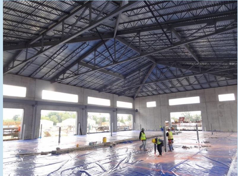
Radiant floor tubing to be installed and then place concrete next week
