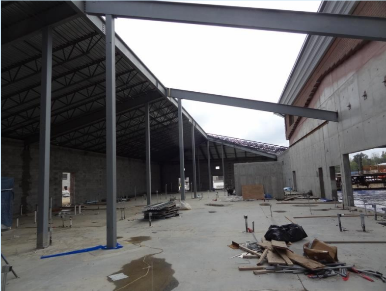
Administrative Area - Will start rest of roof deck now that brick work done to right
