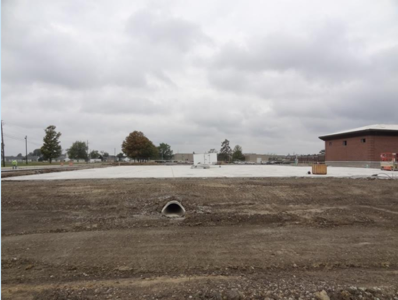
VMF MEP parking
